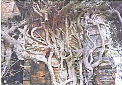
Damage by a banyan tree on Lal Masjid
