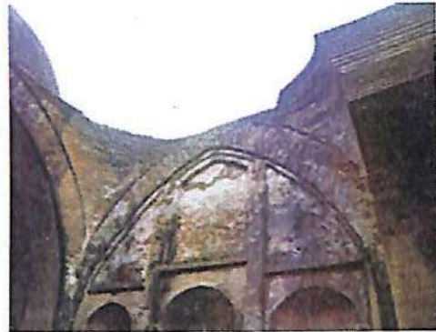
Dome of the Katra Mosque, Murshidabad, might have broken by Earthquake
