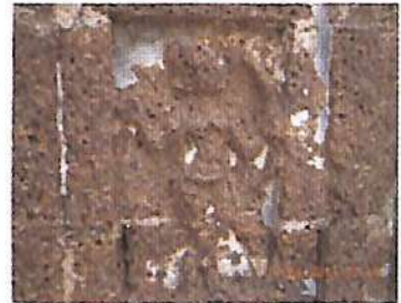
Damaged Terracotta Figure, Radhagobindo Temple, Bishnupur
